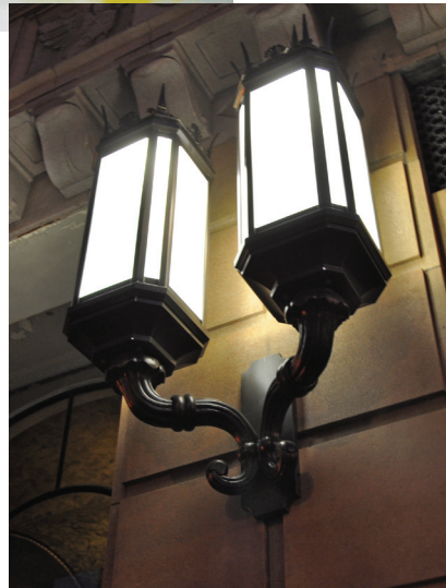
This decorative light by ADG that uses induction technology is installed on the Pershing Square building in downtown Los Angeles.
